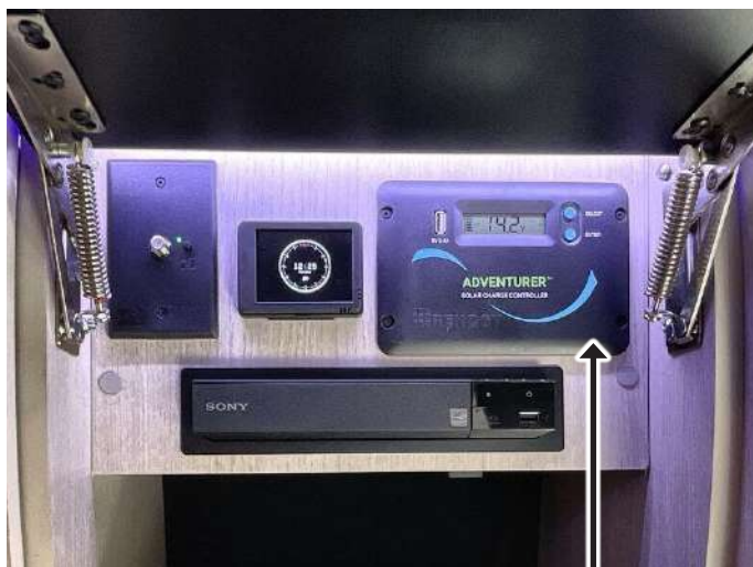
Battery Charger Solar Controller
