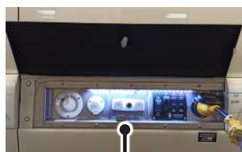
Roadside Utility Compartment
