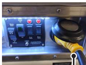
Shore Power Cord Hookup
